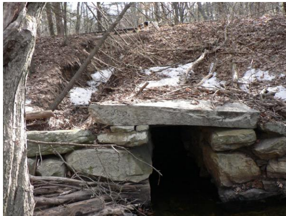
Figure 2: Washed out area above culvert No. 43.89 east of Shepherd's in Townsend
