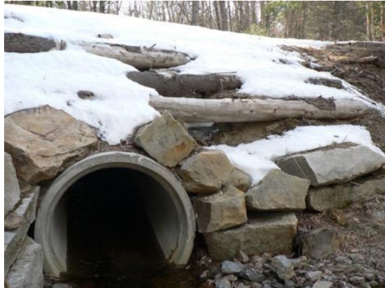
Figure 1: Erosion above culvert No. 42.37 east of Harbor Village
