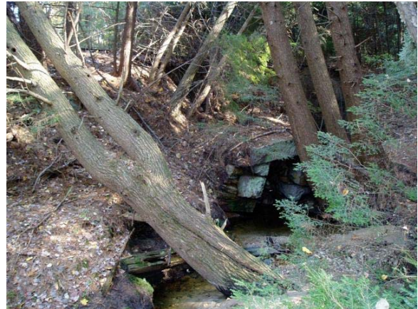
Figure 43: Culvert No. 42.37 Collapsed Culvert
