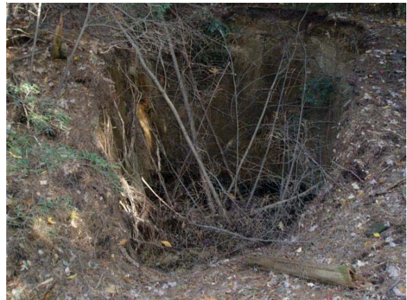
Figure 44: Culvert No. 42.37 Failing Railroad Embankment
